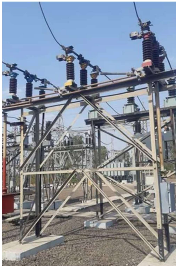
FIG: ISOLATOR USED IN SUBSTATION
