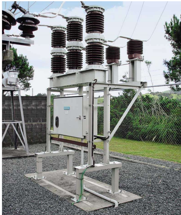
FIG: CIRCUIT BREAKER
