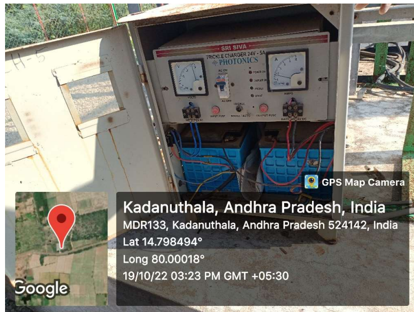
FIG: DC SUPPLY INTERIOR VIEW
