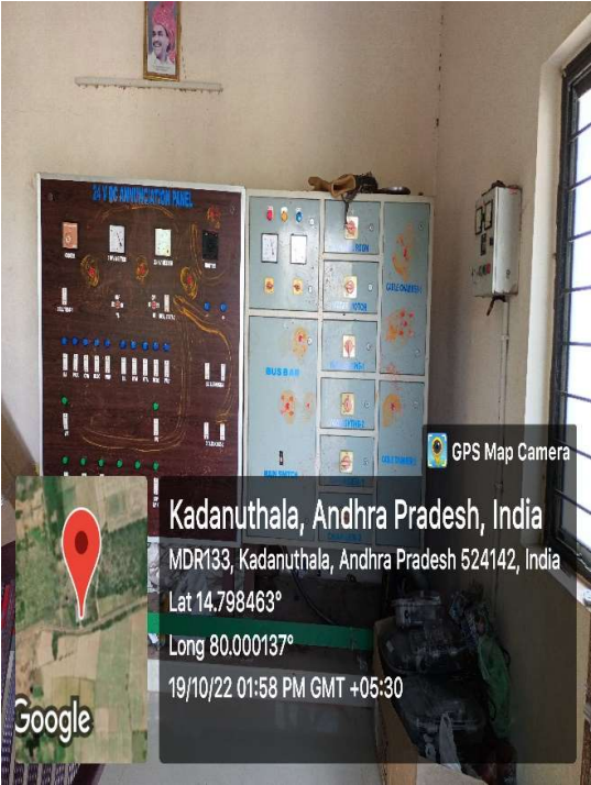
FIG: CONTROL ROOM IN SUBSTATION
