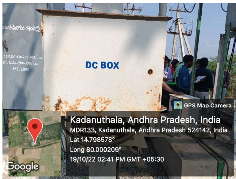
FIG: DC BOX FOR CIRCUIT BREAKER
