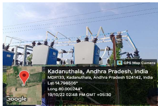
FIG: CAPACITOR BANKING IN SUBSTATION
