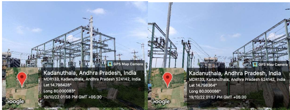
FIG: SUBSTATION YARD FILLED WITH GRAVEL
